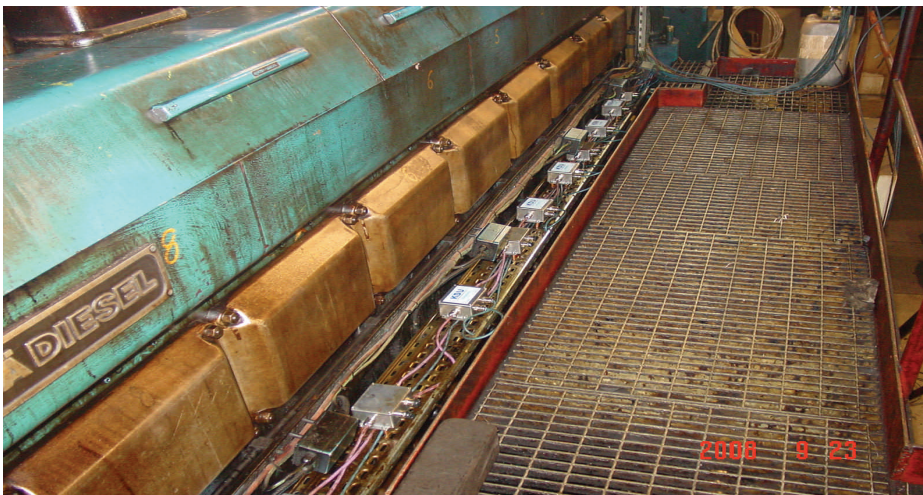
EDS network laying along the side of a Wartsila diesel engine
